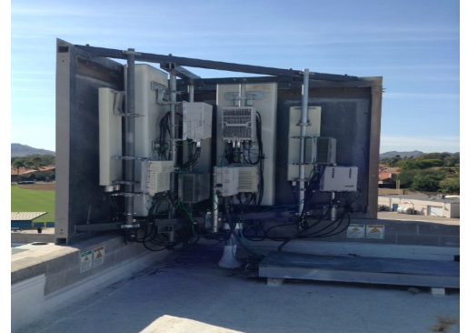
Fig 1 - Antennas at Gym Room (1 of 2 Locations)
