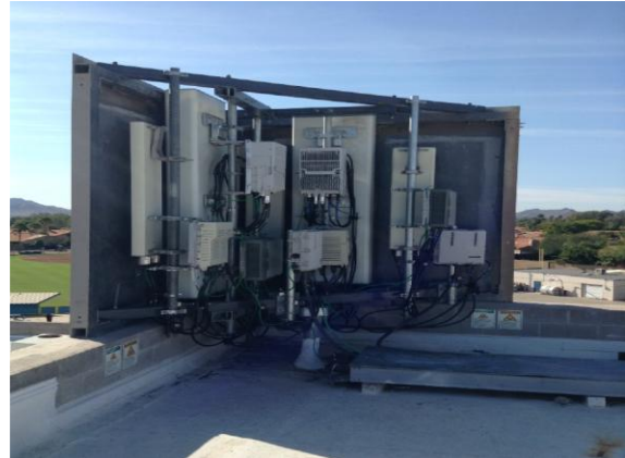
Fig 1 - Antennas at Gym Room (1 of 2 Locations)
