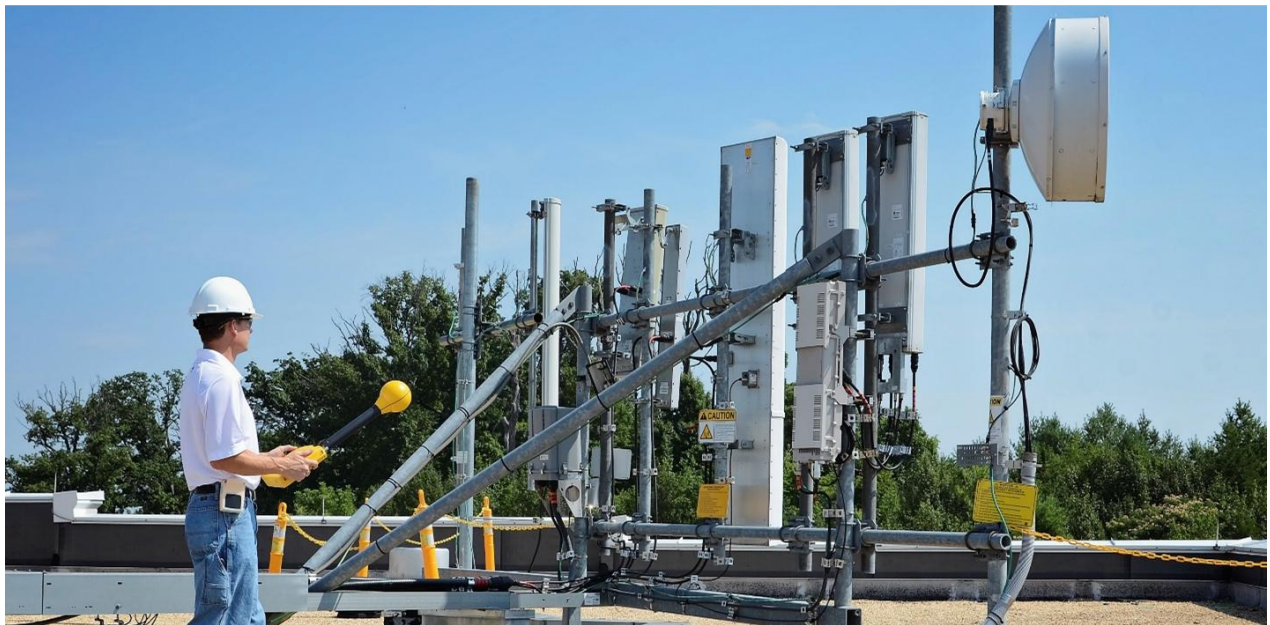
FIG. 4 – PHOTO OF FIELD RF MEASUREMENTS AND SITE AUDIT AT A ROOFTOP WIRELESS SITE IN STERLING, VA
